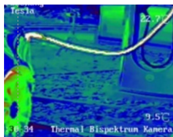
EV Charging Station
