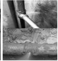
Fire Sprinkler System
