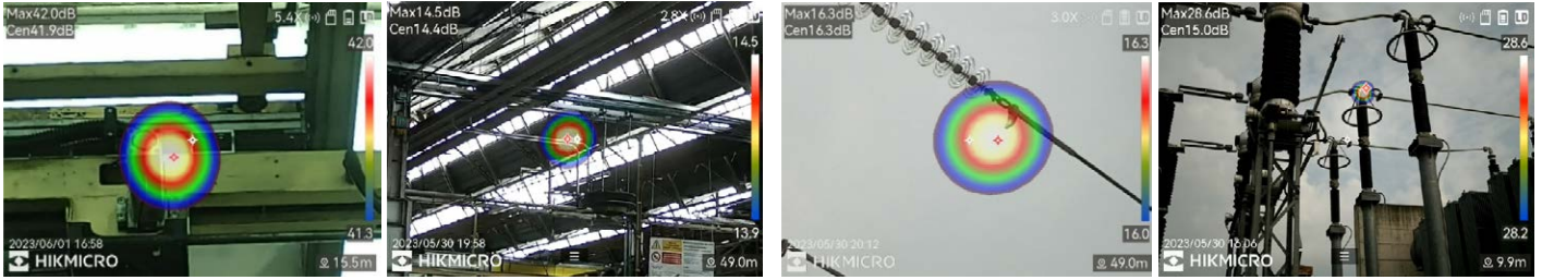
Gas Leak Detection
