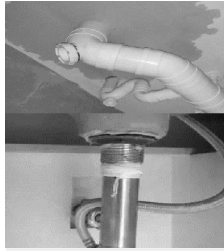
Water Supply Pipe Leakage/ Water Pipe Leakage
