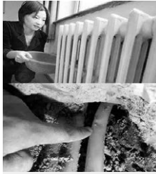
Heating Pipes/ Underfloor Heating Pipe Leaks
